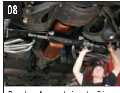
08 The rack was then mounted in position. This gave us the opportunity to check for interference with other components. The instructions warned of possible interference with the motor mount and the factory headers. They were right!
