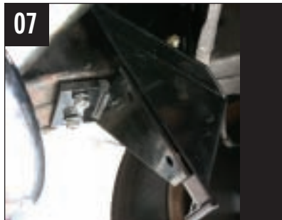
07 Rack mounting brackets were then bolted in place using the factory steering box, assist cylinder, and idler arm attachment points, and were torqued to 35 ft.-lbs.
